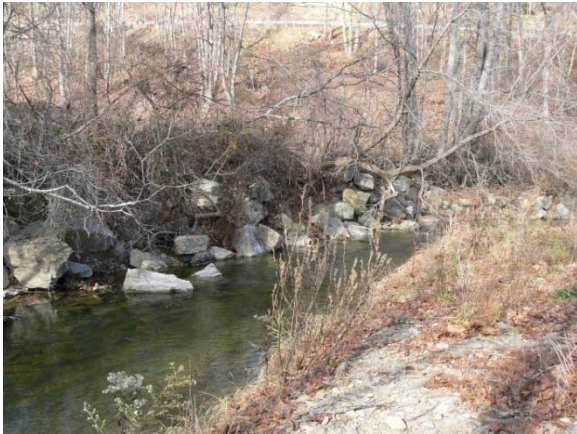
Streambank Erosion, attempts to control bank erosion, and failing riparian zone, at Site FPR-2. (312: 11/19/2008–12:44 pm)
