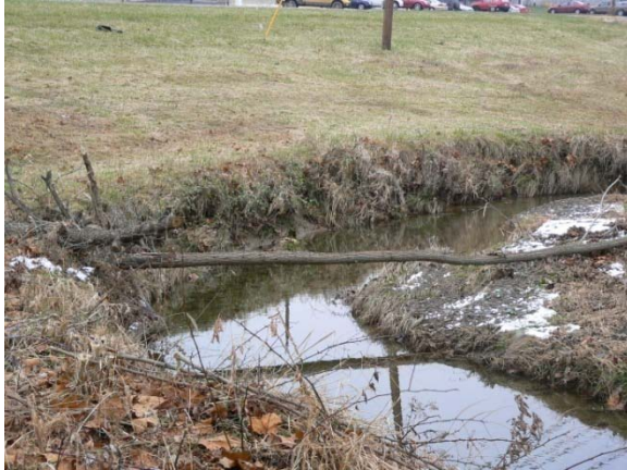
Streambank erosion along Bennetts Run, parallel to Fairfield Road - Site FPR-5. (353: 11/20/2008 – 1:33 pm)
