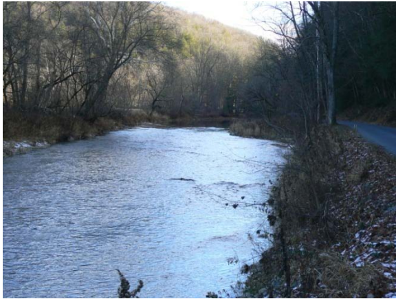
Streambank Erosion threatening Rock Road, on Little Muncy Creek, at Site FPR-8. (314: 11/19/2008 – 1:01 pm)
