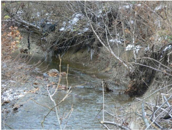
Streambank erosion along Bennetts Run, parallel to Fairfield Road - Site FPR-5. (349: 11/20/2008 – 1:30 pm)
