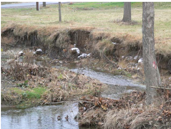
Streambank erosion along Bennetts Run, parallel to Fairfield Road - Site FPR-5. (355: 11/20/2008 – 1:34 pm)
