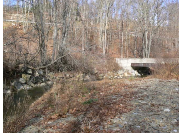
Streambank Erosion, and failing riparian zone, at Site FPR-2. (313: 11/19/2008 – 12:44 pm)
