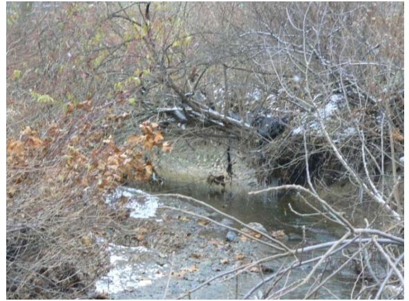
Streambank erosion along Bennetts Run, parallel to Fairfield Road - Site FPR-5. (350: 11/20/2008 – 1:30 pm)
