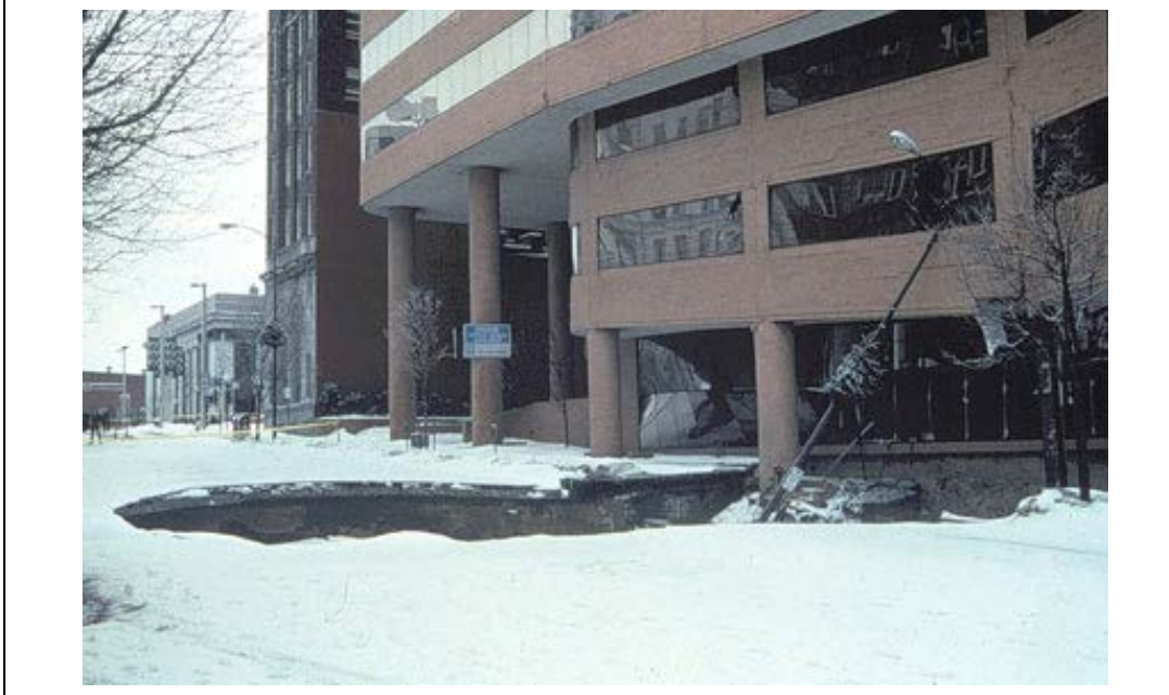
Figure 4.3.6-2 Sinkhole at Corporate Plaza Building in Allentown, Lehigh County, PA in February 1994 (Photography by William E. Kochanov – DCNR, 2009)
