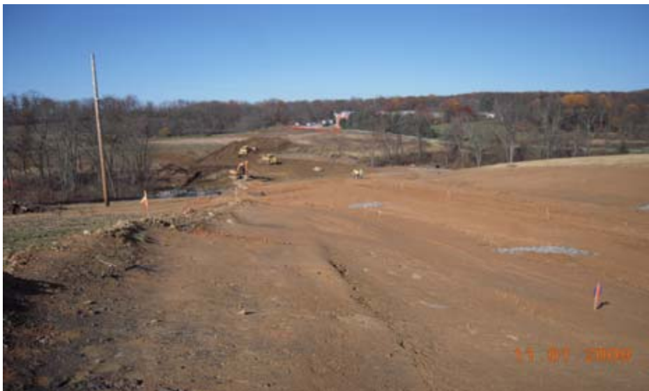
Construction of Alexander Drive in Muncy Township for future economic development of surrounding properties
