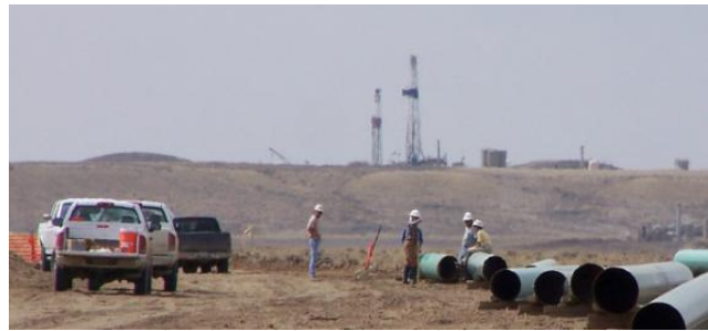
Figure 11: Workers lay pipelines among drilling rigs in Sublette County, WY. Circa Summer 2006
